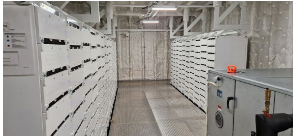
Battery room, or the 'holy of holies'. Here we see all the battery packs that power the MF Suløy.
